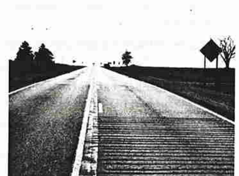
f) Rumble strips and advance signing add to cues to drivers approaching from the north.
