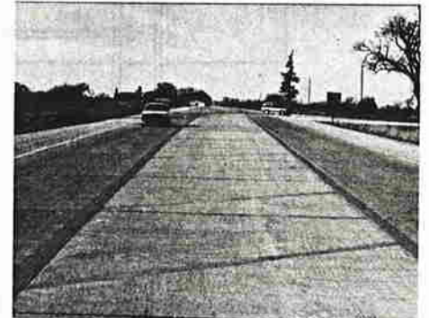
c. Painted channelization provides separation of opposing flows, protection for the west to north left turn lane, and visual notice of the intersection.
