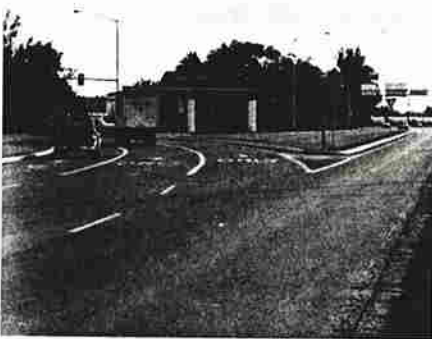
(d) Through traffic onto Exposition Drive proceeds on a smooth, flat horizontal curve. Note the blunt approach end of the "right" turn lane island nose.
