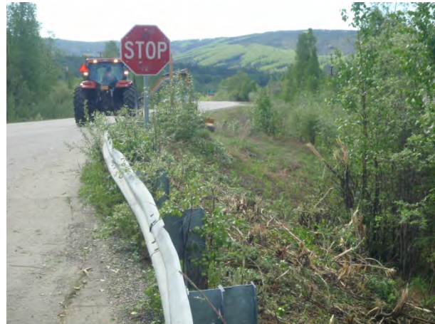
Photograph 2: Mechanical control of Zones 1 and 2 unable to address guard rail vegetation.
