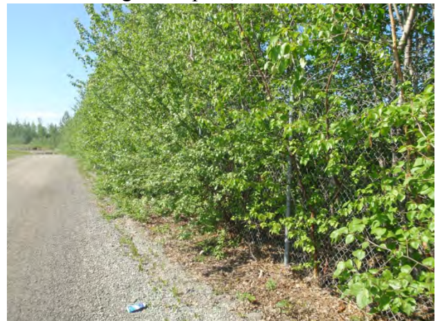
Photograph 5: Fast-growing woody vegetation damaging perimeter airport fence lines.
