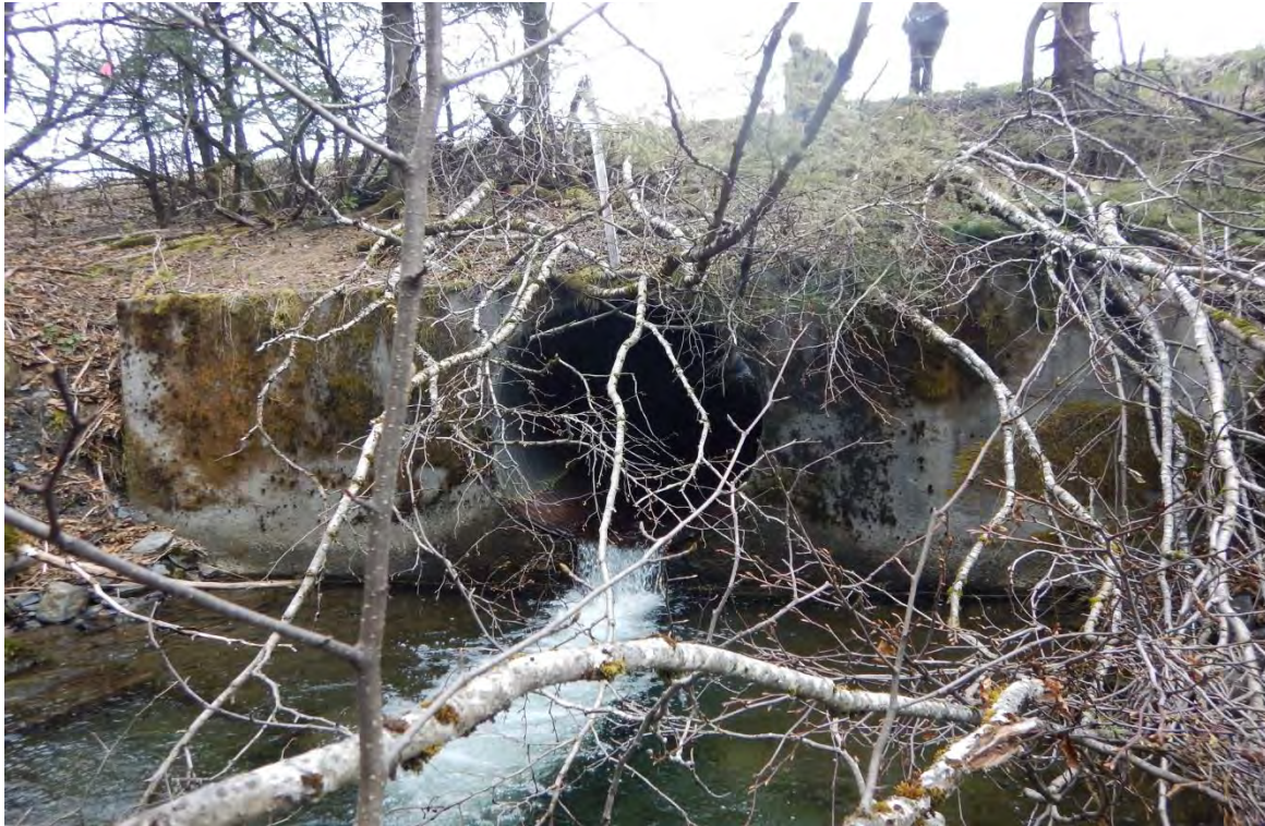
Figure 4. Perched culvert outlet located at the south end of the runway.
