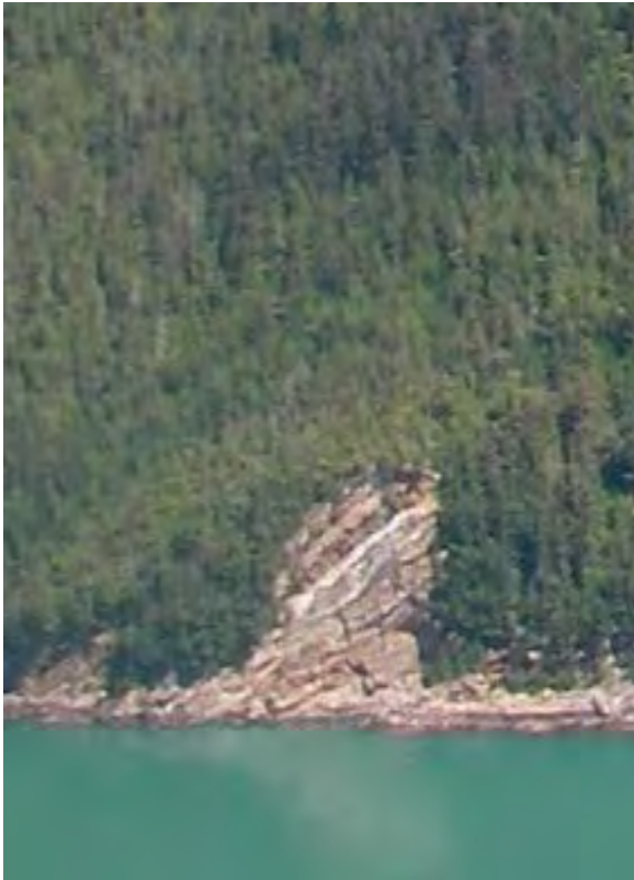
RF08. View east/upslope at rockfall hazard.
