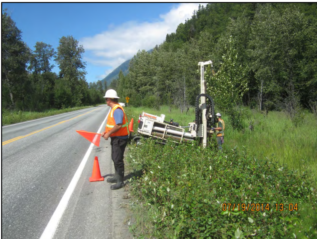
Photograph 2 – Flaggers alerted oncoming traffic when drilling activities were near road shoulders. View to the northwest.
