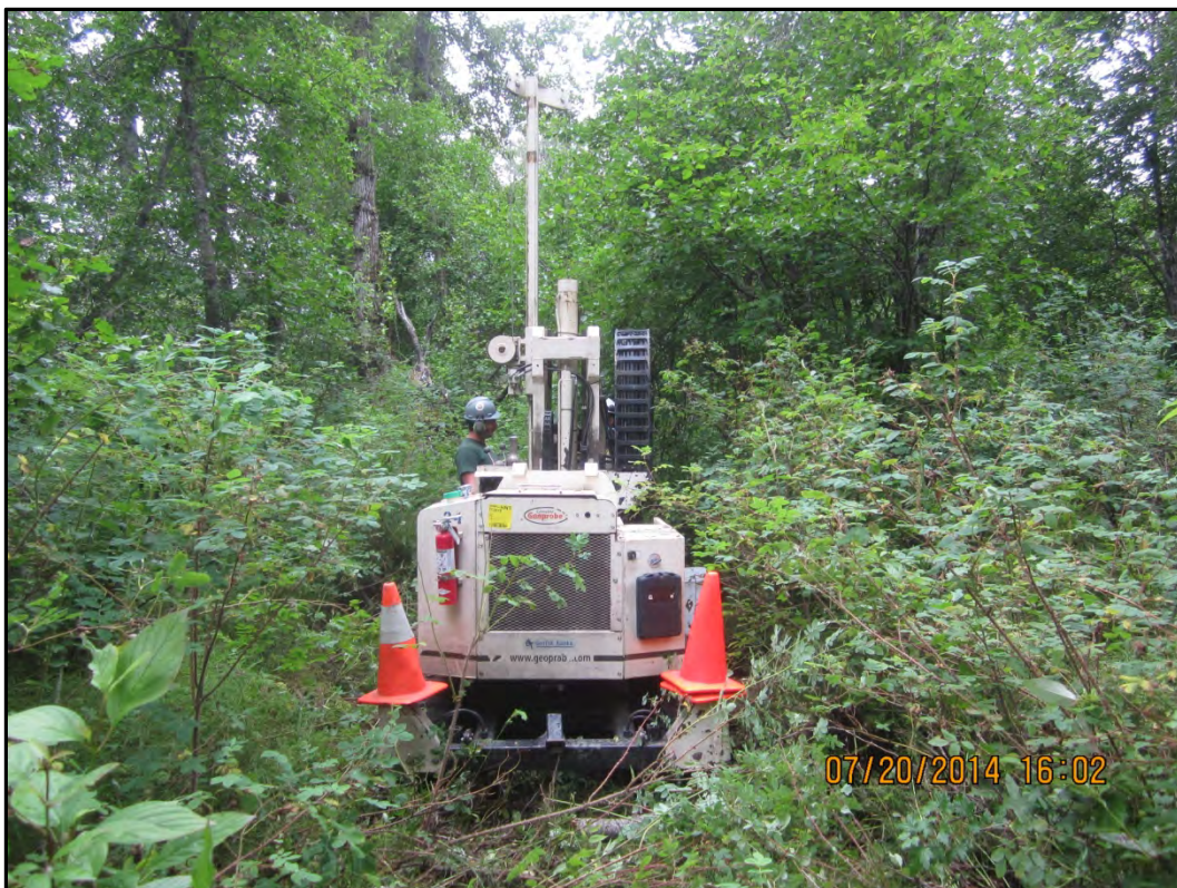
Photograph 4 – Drill rig set up on boring 17-BH21 on the south side of the Haines Highway. View to the southwest.
