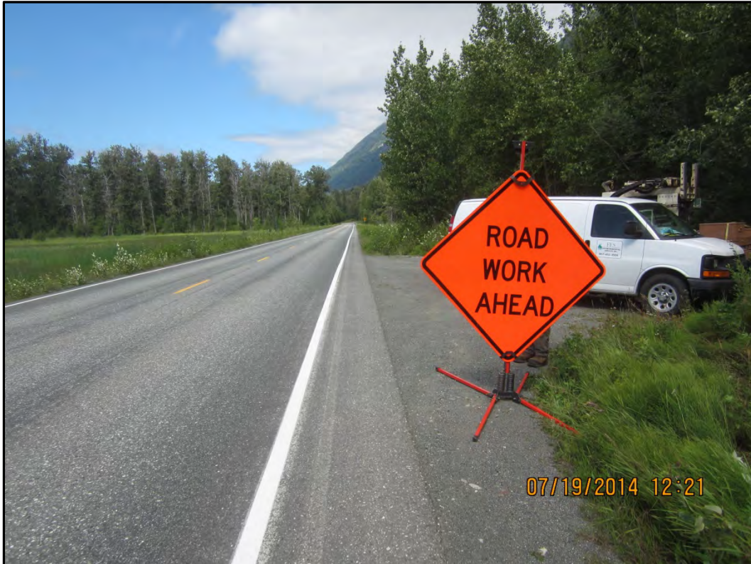
Photograph 1 – Road signs were put at both ends of the Haines Highway (in working areas) prior to starting drilling activities. View to the northwest.
