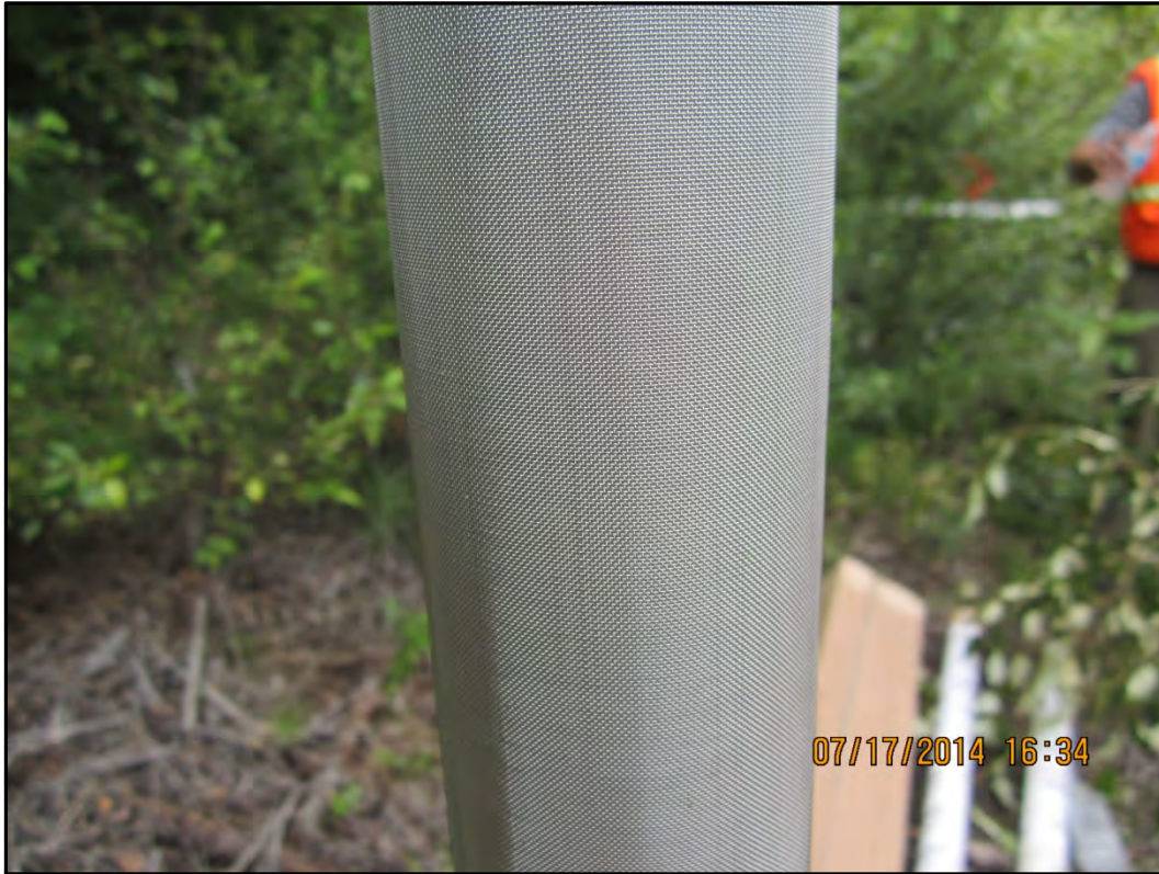
Photograph 47 – 1.5" Pre-Pack PVC with stainless steel mesh well screen was used in all wells.
