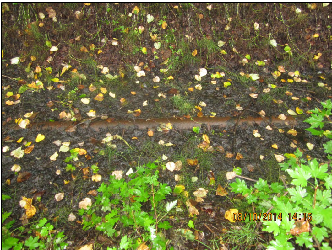
Photograph 12 – Exposed (above ground) Haines-Fairbanks Pipeline. Surface water was 1-2 feet shallower in mid August 2014 compared to mid July 2014.
