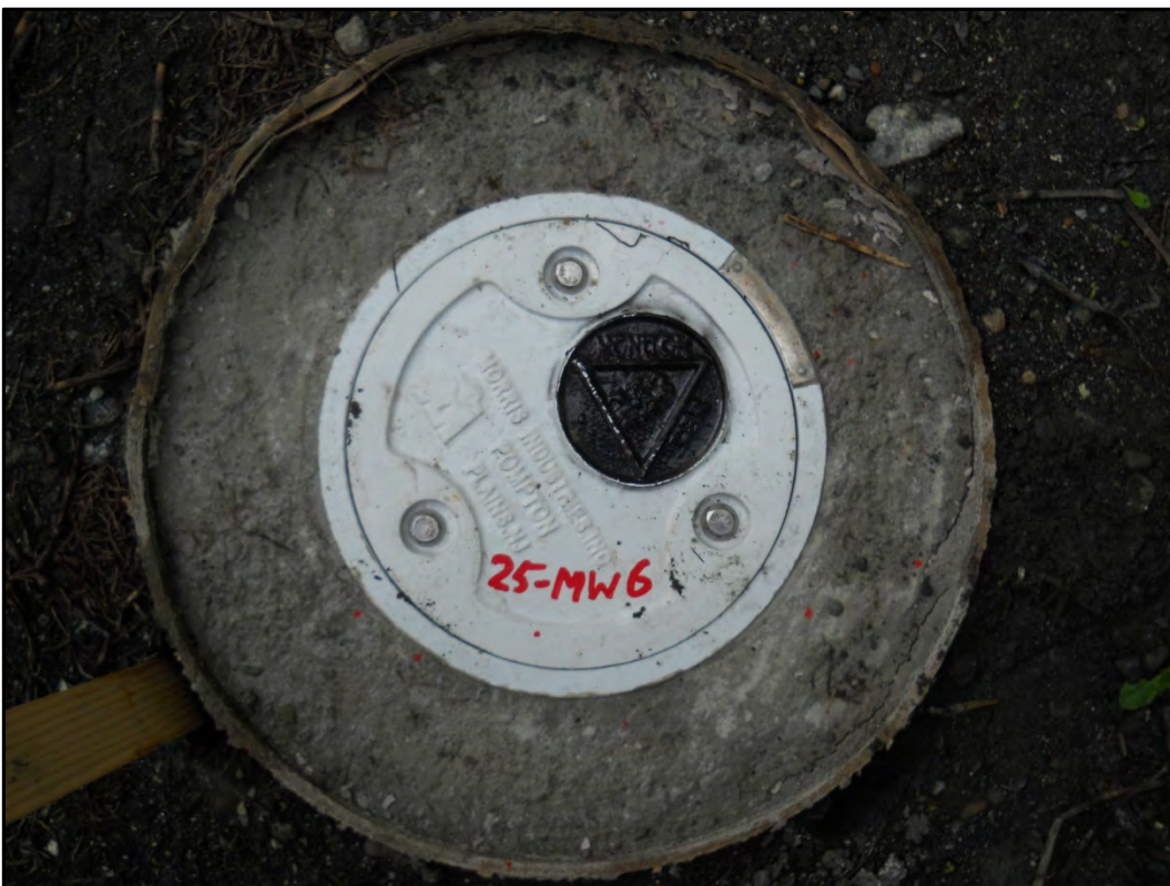
Photograph 50 – Closeup view of flushmount well 25-MW6.
