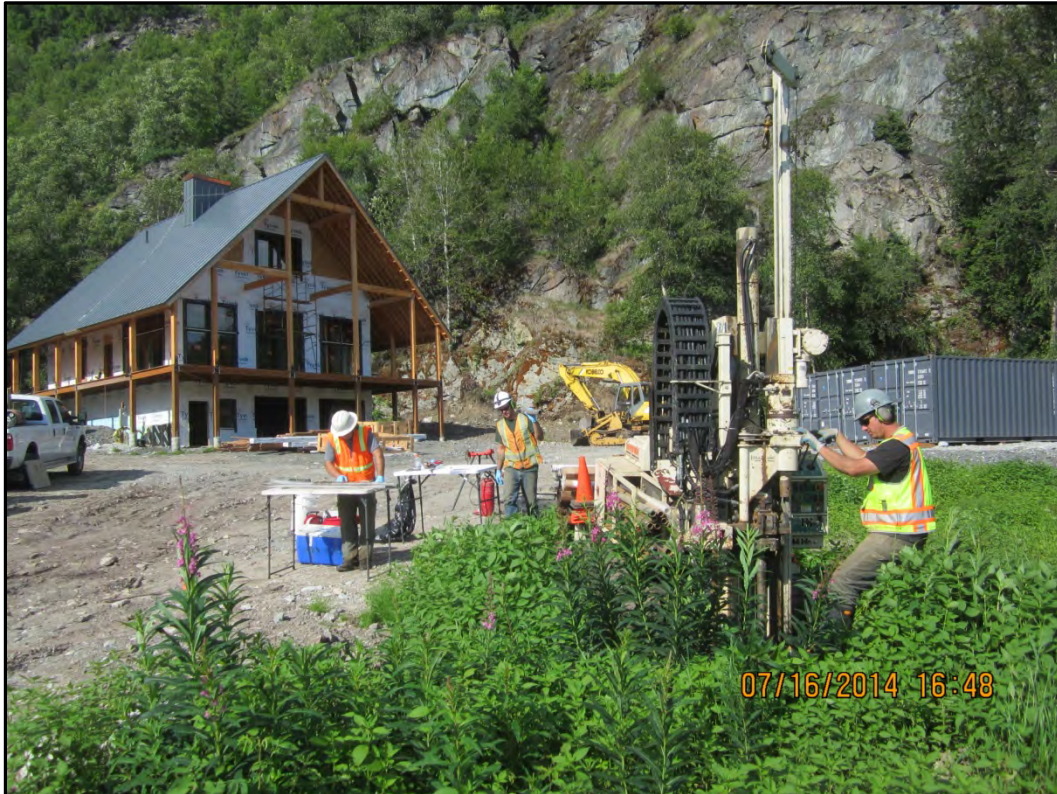
Photograph 21 – Geotek Alaska drilling 19-BH12/19-MW2. Note: New house under construction in background. View to the north-northeast.
