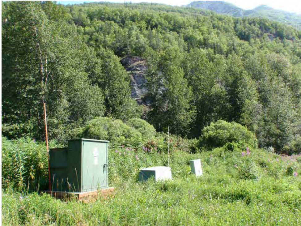
PMP 19.5– Utility Boxes Near Where Fuel Odors were Reportedly Identified (Photo Taken from along Haines Highway – Looking Northeast)
