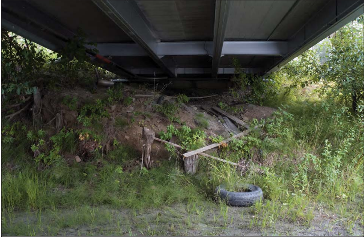
Figure H-10. Pilings from the 1943 bridge (SKG-549) in place beneath the southern end of the current bridge.
