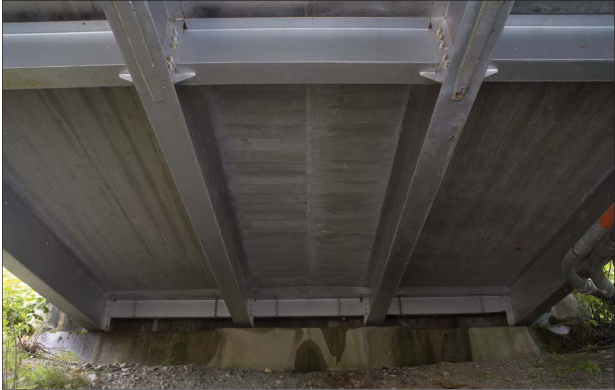
Figure H-16. Form marks on the underside of the concrete roadway showing the sequence of the concrete deck pour.
