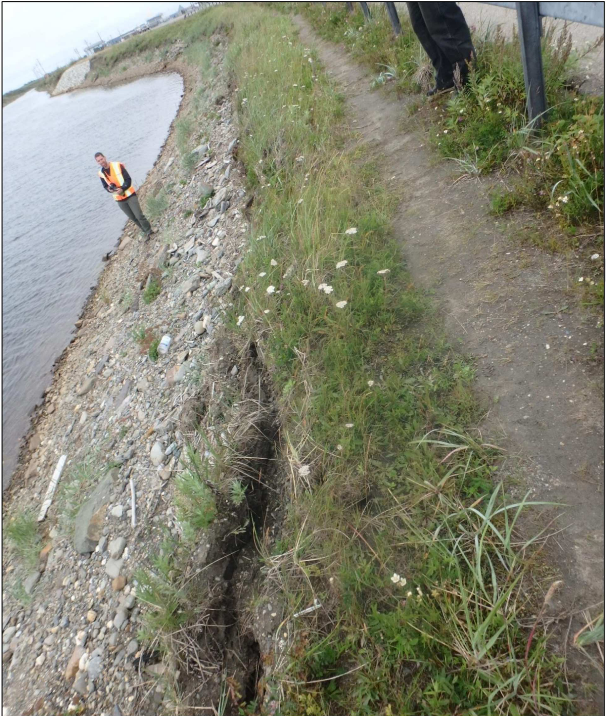
Figure 2. Tension crack at top of Snake River bank, upstream of new bridge. PDC Engineers photo.
