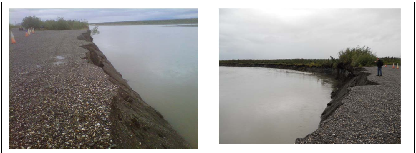
Figure 5: Bank Erosion August 2012 Orange cones set along east side of Pit Road. (Left) looking upriver from Point C (Right) looking downriver from Point B
